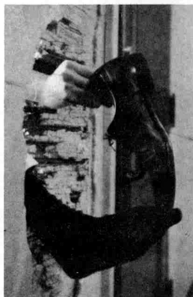
BEFORE AND AFTER . . . Last week The Acorn showed a picture of the hole in the boys' lavatory on the second floor of the old building. As a comparison of this picture to that shown last week reveals, the large termites responsible for the damage made considerable progress. Fortunately, however, the room was boarded up last week.
